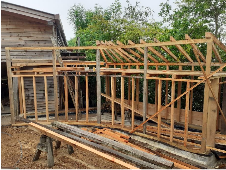
Photo 5 Building a small timber building with a curved front from scratch (Photo Jonas Brandl)
